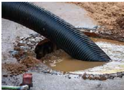
Collapsed Sewer Pipelines
